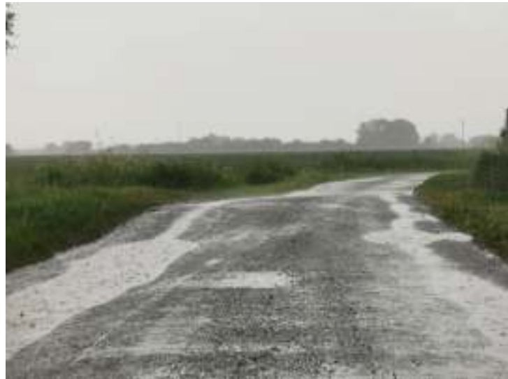
Figure 60: The slight rise visible in the centre of the picture represents all that remains of the line of High Bank as it goes across Marsh Lane, Grainthorpe.
